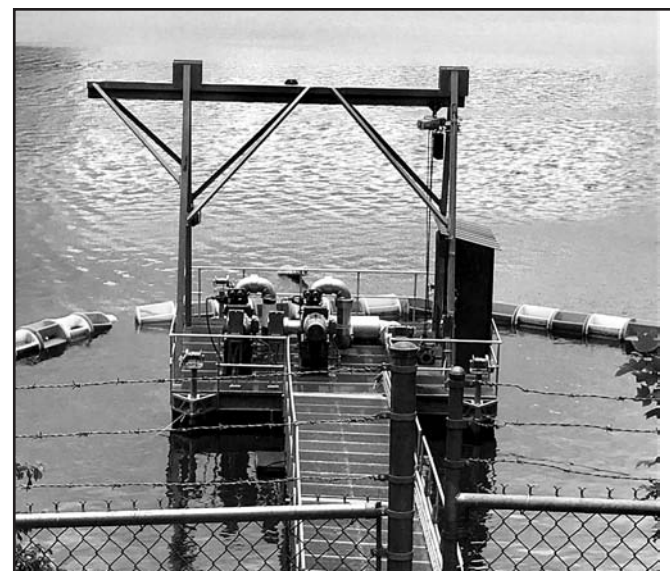
The intake pumps in Lake Chatuge, out at the water treatment facility in Hiwassee.
